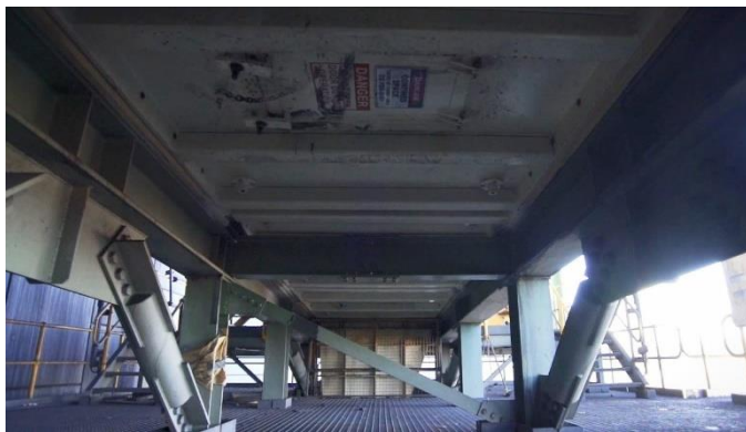
General arrangement of feeder "underbelly" showing newly installed modules.
